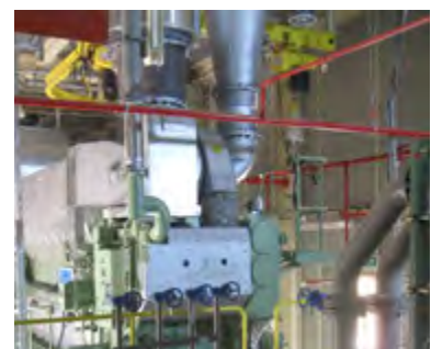
Inside view of Enclosure(Pre-fabricated type)
