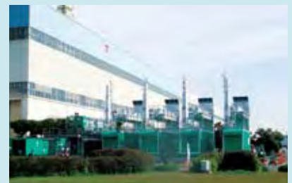
J-Project 5.6 MW PPS in Japan (HYUNDAI - HiMSEN 9H21/32 x 4 Sets)
