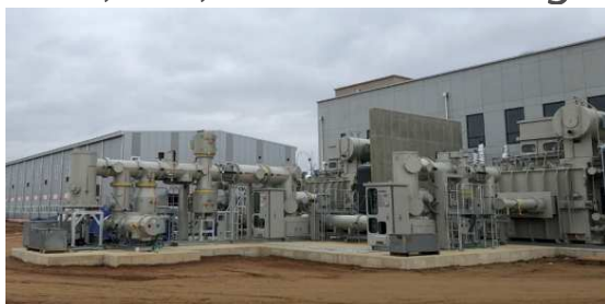
TR, GIS, Control Building
